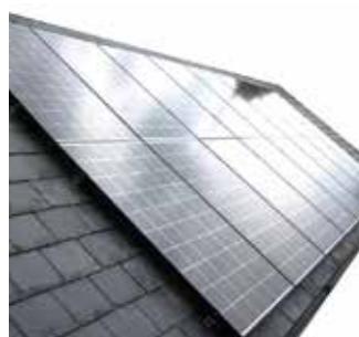
Solar PV panels
